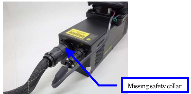
The safety collar is missing at the laser head connection.
